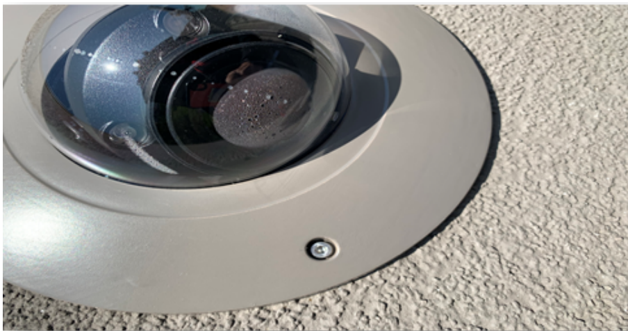
Figure 1-6 Moisture inside the camera
