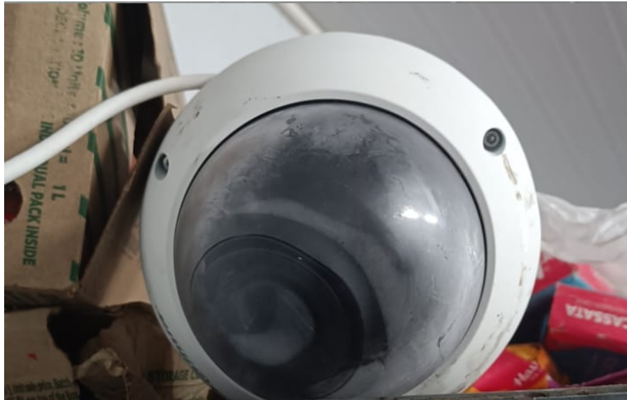
Figure 1-7 Moisture on the surface
